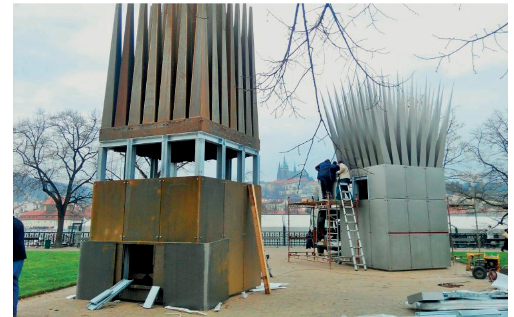
040 Monument to Jan Palach (The House of a Suicide and The House of the Mother of the Suicide), John Hejduk, arch. Pavla Melková, Miroslav Cikán (2016) [Prague 1, Jan Palach Square/Alšovo Embankment]
